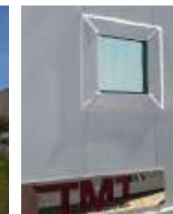
Window for load inspection
